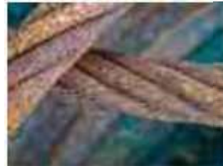
RUST/DISCOLORATION Cable is rusty, orange, weathered or dull
